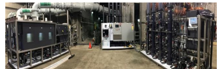
York River Pilot Plant
